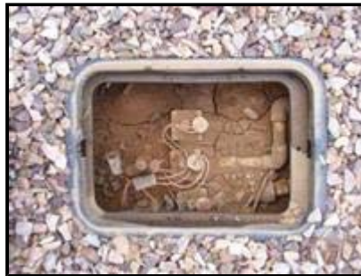
Front yard valves
