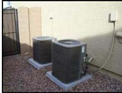
Exterior compressor/condenser units
