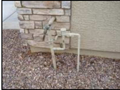
main water valve
