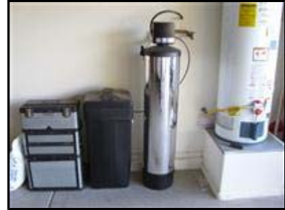
water heater & conditioner
