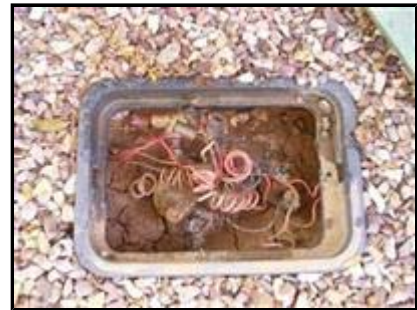
Rear yard valves
